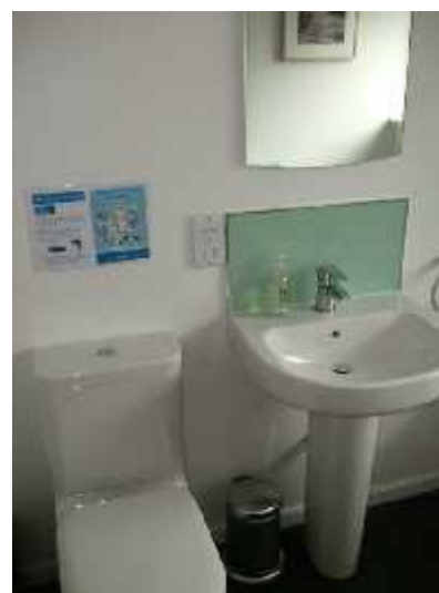
Bathroom sink and toilet
